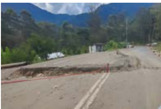
Subsidence damage due to a major landslide
