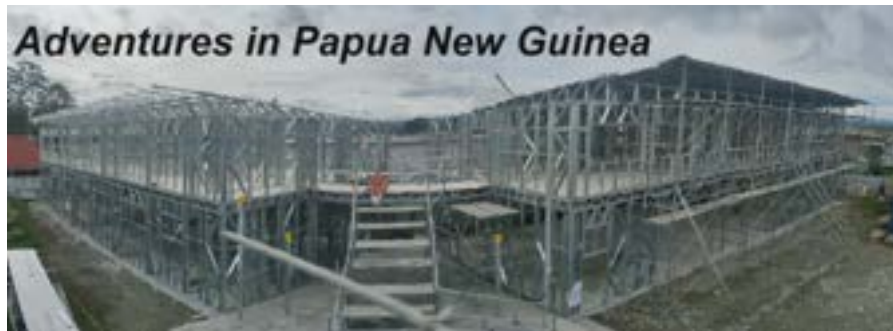
Caroline sits in the middle of the framework of our new Motel & Conference facility currently under construction
